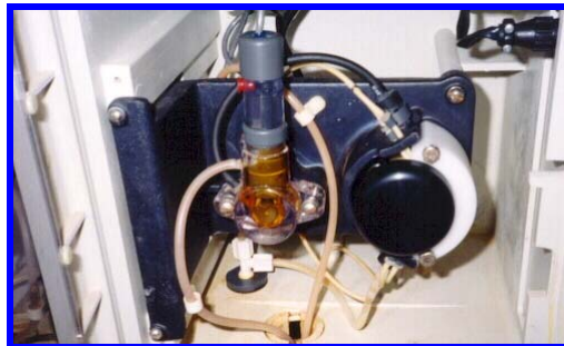
Inside Chlorine Residual Analyzer Sample Cell and Reagent Pump
